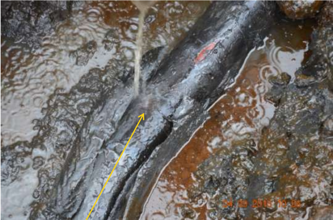
Close up: Spill due to corrosion on 4" Cawthorne Channel 2 Well 29T flowline at Mbiama. Picture was taken during Joint Investigation of 4 th September 2013.
