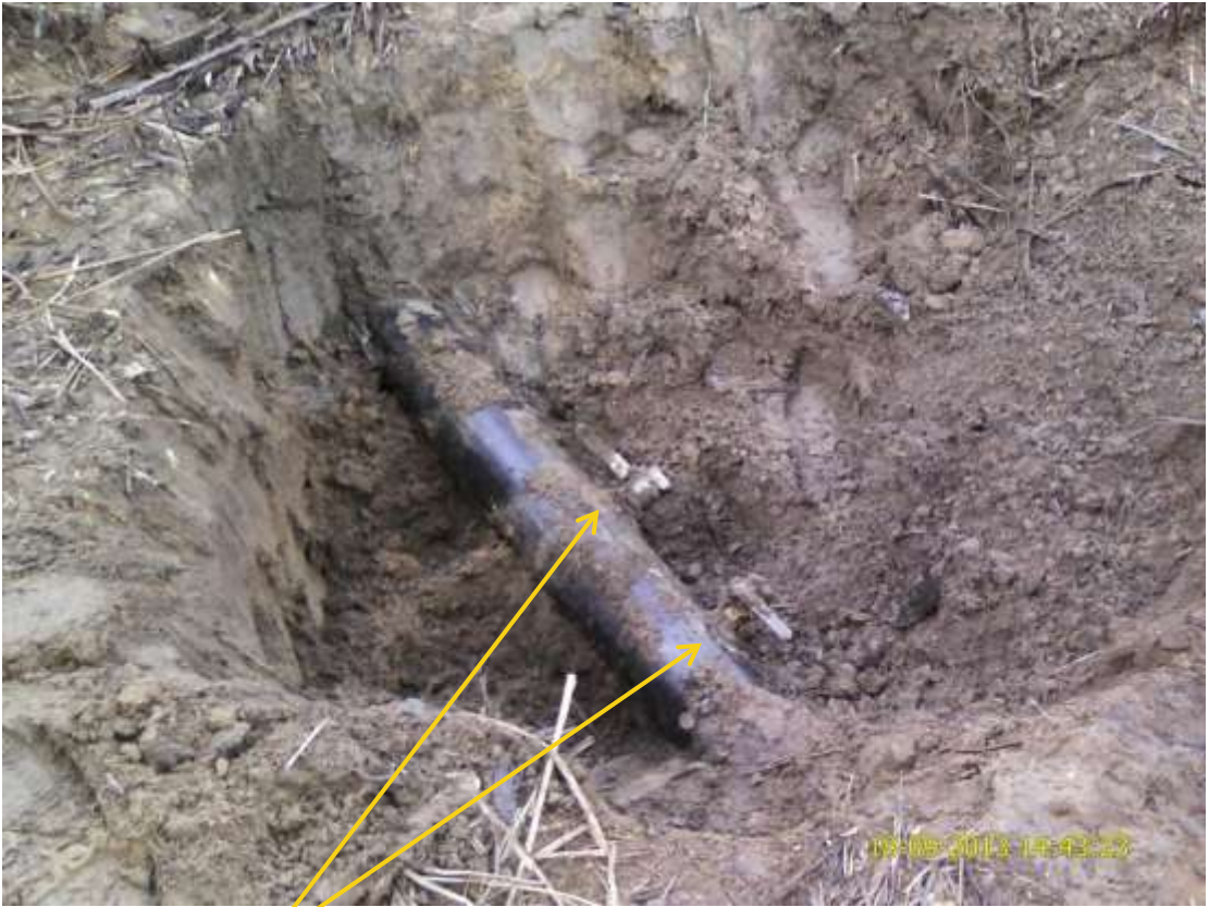
Close up: Illegal fittings on 6" Imo River 59T flowline at Igiriukwu. Picture was taken during Joint Investigation of 18 th September 2013.
