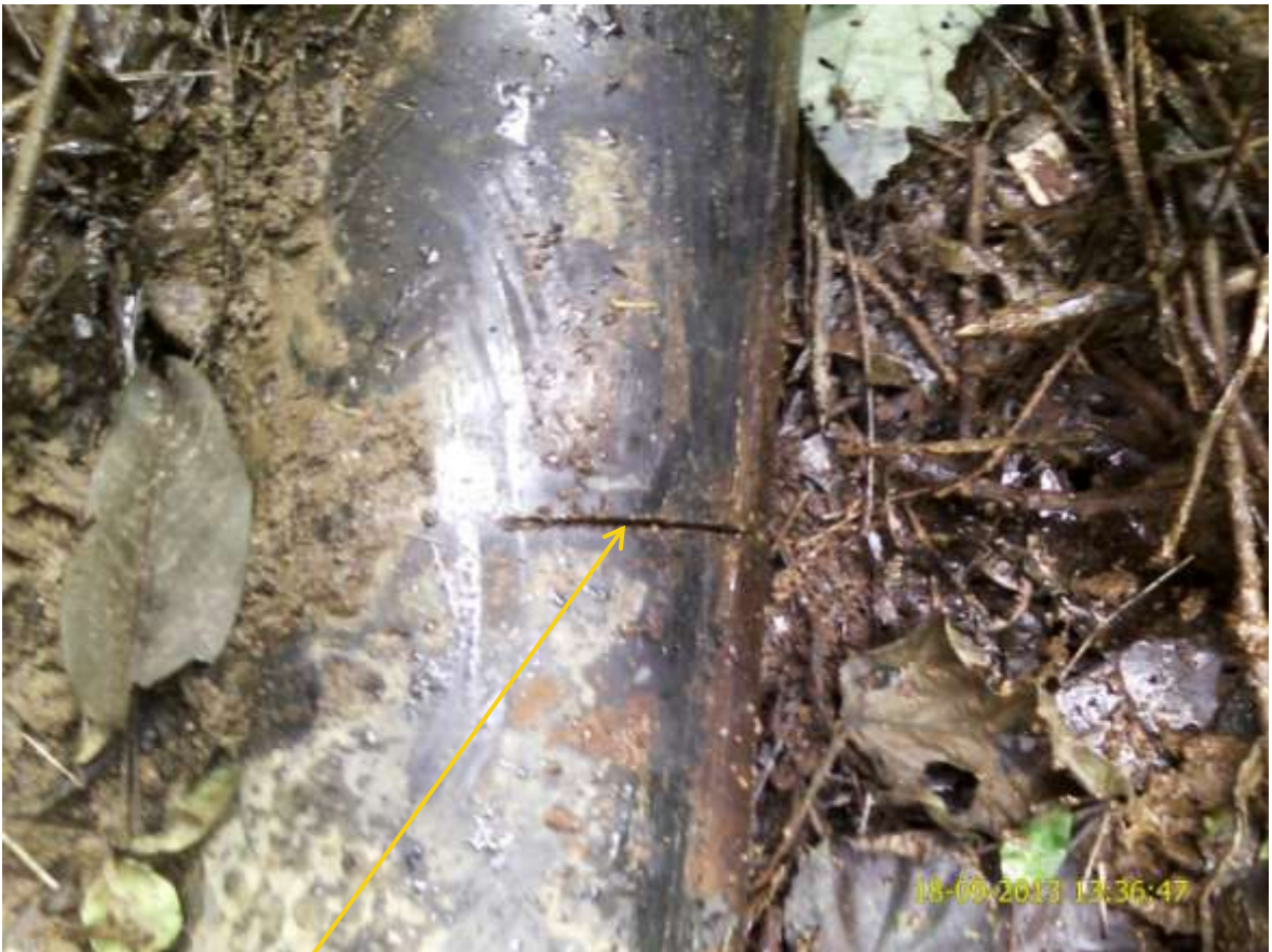
Close up: Hacksaw cut on 6" Imo River1 30L flowline at Igiriukwu. Picture was taken during Joint Investigation of 18 th September 2013.
