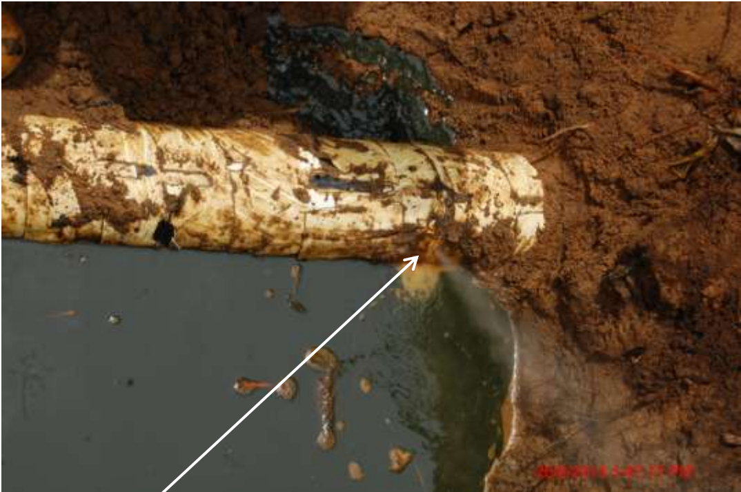
Close up: Hacksaw cut on 4" Ubie Well 5L flowline at Idu Ekpeye. Picture was taken during Joint Investigation of 26 th September 2013.
