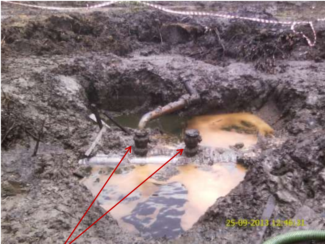
Close up: Illegal fittings on 28" Bomu-Bonny pipeline at Oloma. Picture was taken during Joint Investigation of 25 th September 2013.
