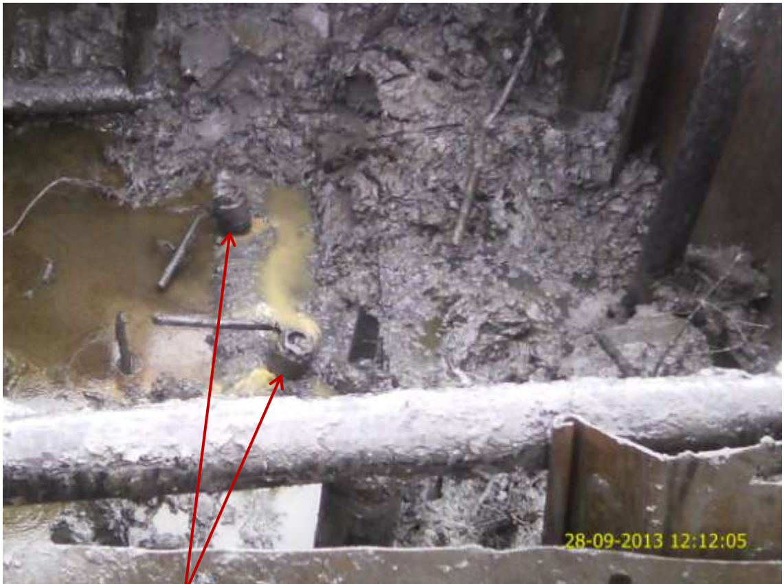
Close up: Illegal fittings on 24" Bomu-Bonny Trans Niger Pipeline at Okolo Launch. Picture was taken during Joint Investigation of 28 th September 2013.
