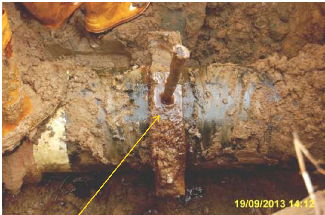
Close up: Illegal fitting on 12" Imo River1 – Ogale pipeline at Umuololo/Owaza. Picture was taken during Joint Investigation of 19 th September 2013.
