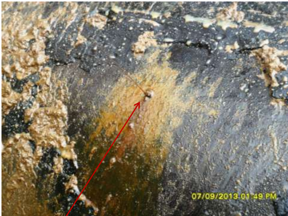
Close up: Drilled hole on 24" Nkpoku-Bomu pipeline at BDere. Picture was taken during Joint Investigation of 7 th September 2013.
