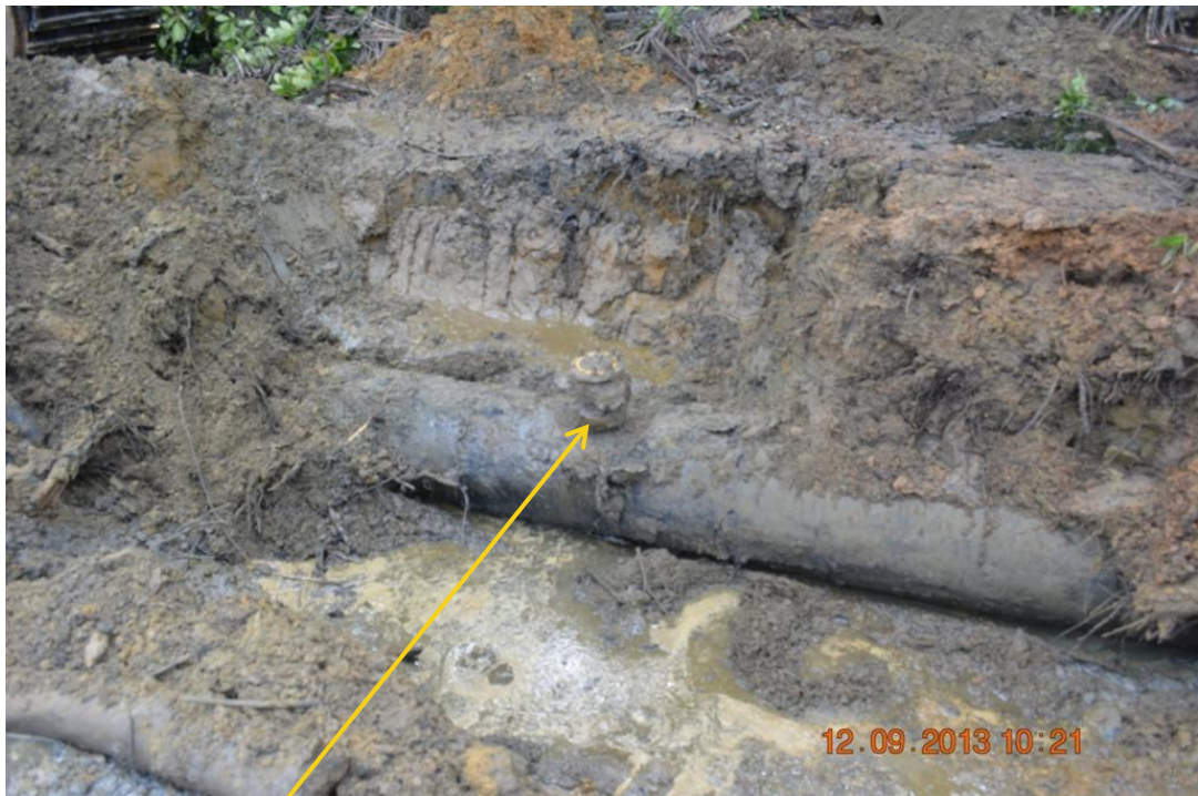
Close up: Illegal fitting on 20" Otumara-Escravos trunkline at Adjudaibo. Picture was taken during Joint Investigation of 12 th September 2013.
