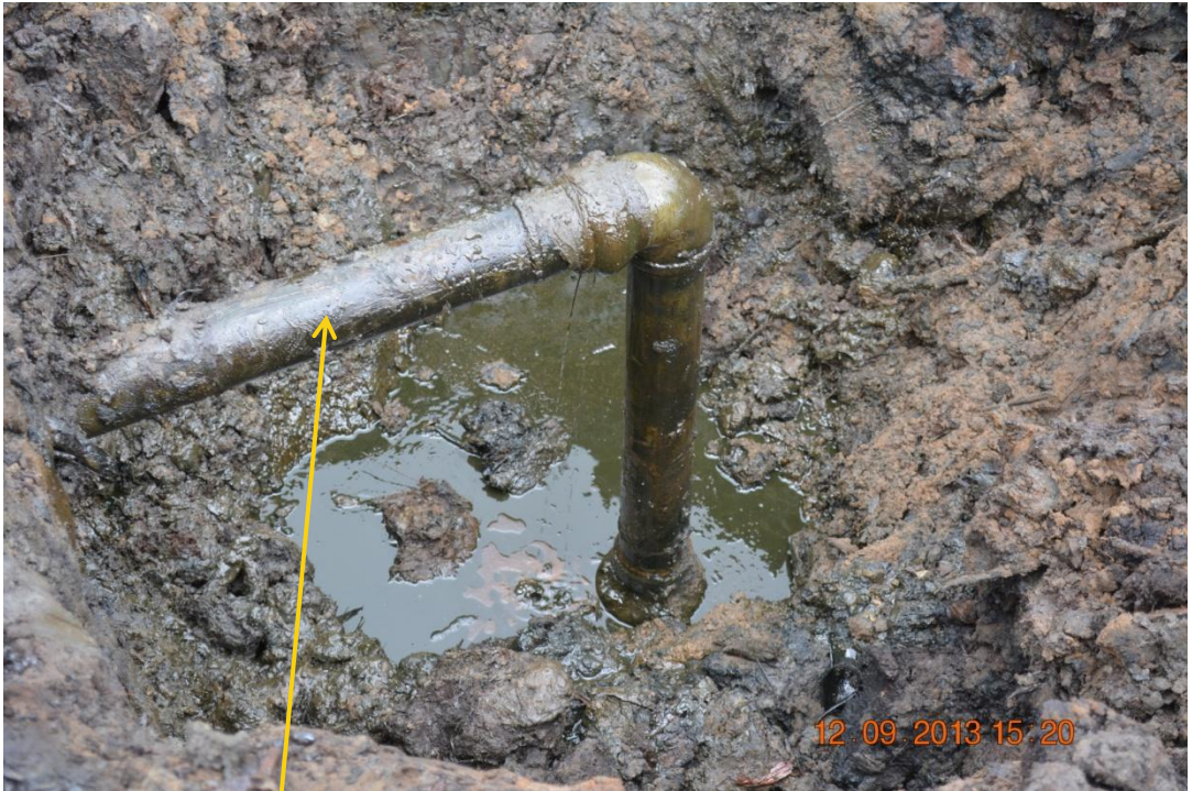
Close up: Illegal fitting on 20" Otumara-Escravos trunkline at Adjudaibo. Picture was taken during Joint Investigation of 12 th September 2013.
