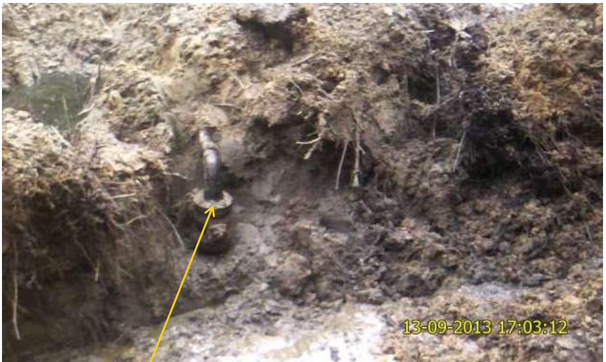
Close up: Illegal fitting on 20" Otumara-Escravos trunkline at Adjudaibo. Picture was taken during Joint Investigation of 13 th September 2013.
