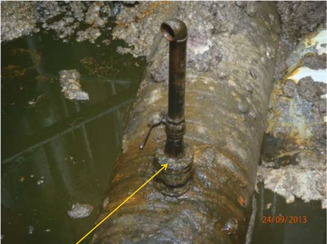
Close up: Illegal fitting on 30" Nembe Creek Pipeline at Krakama. Picture was taken during Joint Investigation of 24 th September 2013.
