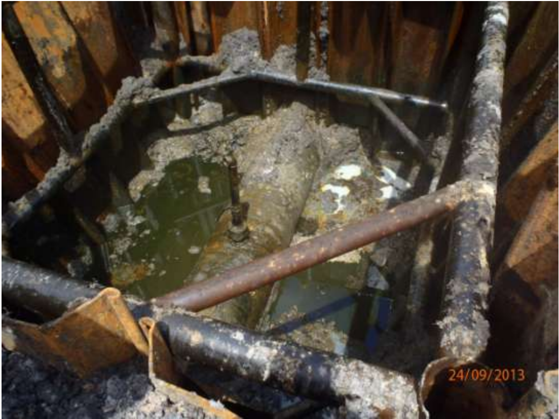
Overview: Spill point within cofferdam on 30" Nembe Creek Pipeline right of way at Krakama. Picture was taken during Joint Investigation of 24 th September 2013.
