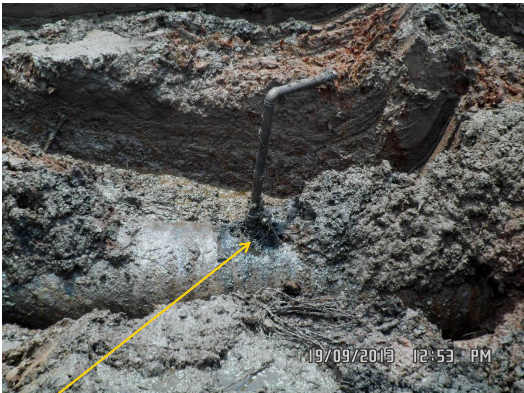
Close-up: Spill due to Illegal fitting on 28" Bomu - Bonny Pipeline at Bodo West . Picture was taken during Joint Investigation of 19 th September 2013.
