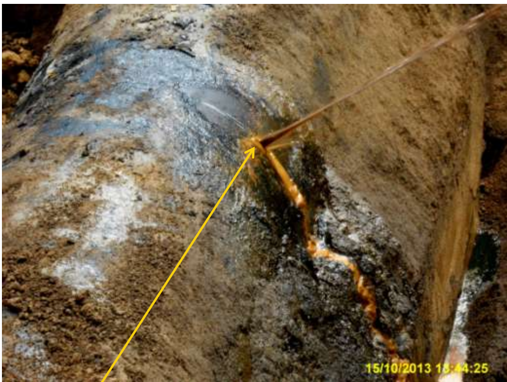
Close-up: Hacksaw cut on 28" Trans Niger Pipeline (near Patrick Waterside manifold) at Bodo-city. Picture was taken during Joint Investigation of 15 th October 2013.
