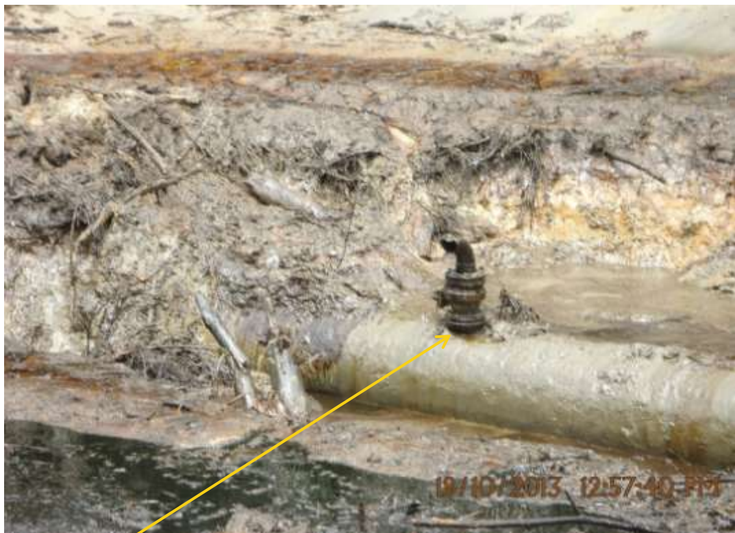
Close up: Spill due to Illegal fitting on 20" Otumara-Escravos Pipeline at Ugboegungun Picture was taken during Joint Investigation of 19 th October 2013.
