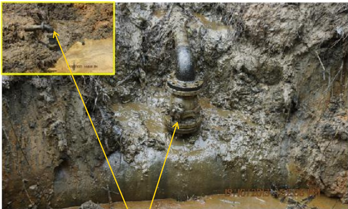
Close up: Spill Points 1 & 2 - Illegal fittings 20m apart on 20" Otumara-Escravos pipeline at Ogidigben. Picture was taken during Joint Investigation of 19th October 2013.
