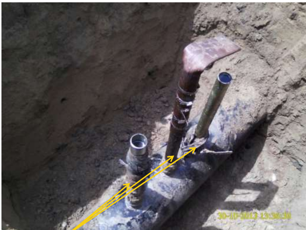
Close-up: Illegal fittings on 12" Imo River – Ogale Pipeline at Okohia. Picture was taken during Joint Investigation of 30th November 2013.
