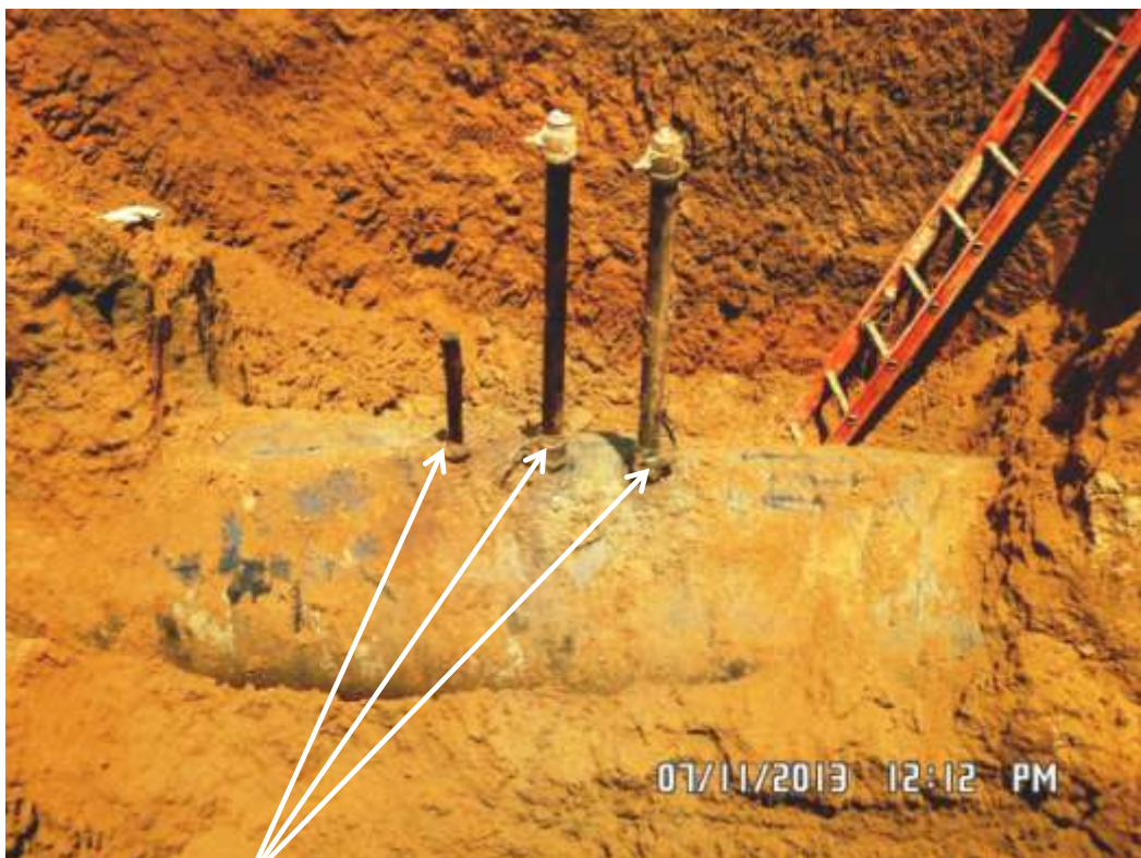
Close-up: Illegal fittings on 36" Rumuekpe-Nkpoku Trans Niger Pipeline at Omuigwe-Aluu. Picture was taken during Joint Investigation of 7 th November 2013.
