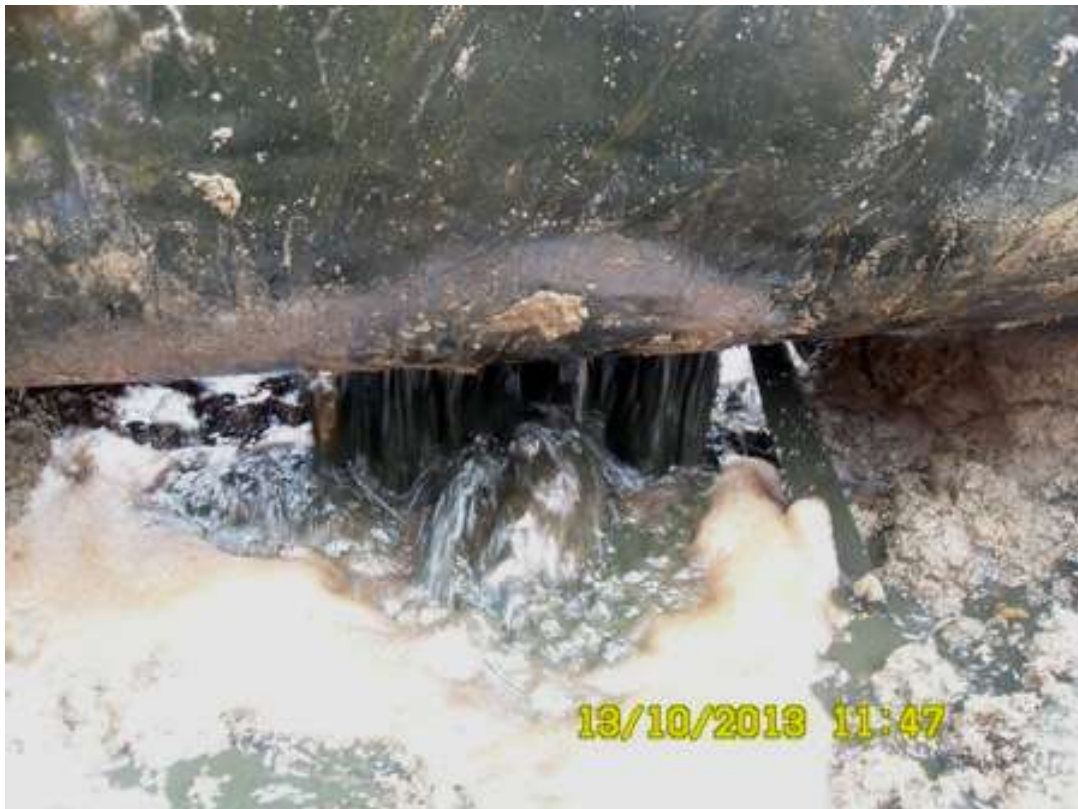
Close up: Spill due rupture of 24" Nkpoku – Bomu Pipeline at Nonwa. Picture was taken during Joint Investigation of 13 th October 2013.
