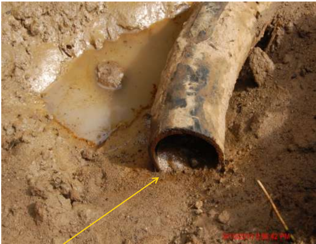
Close up: Missing flowline on 4" Imo River Well 53L/56L Flowline at Etitioha-lpu . Picture was taken during Joint Investigation of 9 th October 2013.
