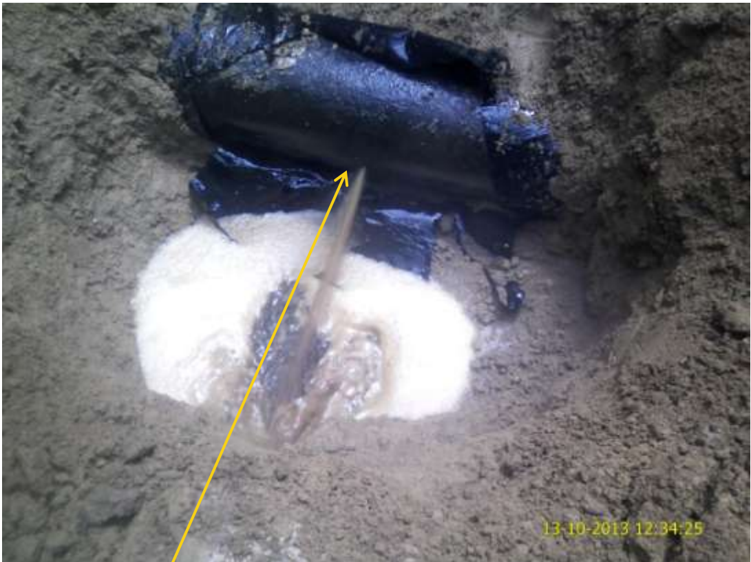
Close up: Spill due to corrosion on 6" Obigbo North – Ebulu pipeline at Obolo. Picture was taken during Joint Investigation of 13 th October 2013.
