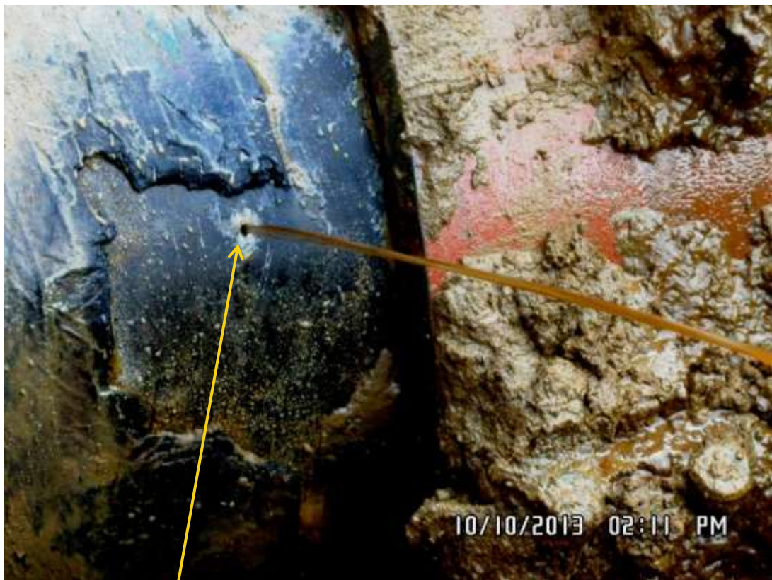
Close up: Drilled hole on 24" Nkpoku-Bomu pipeline at B-Dere. Picture was taken during Joint Investigation of 10 th October 2013.
