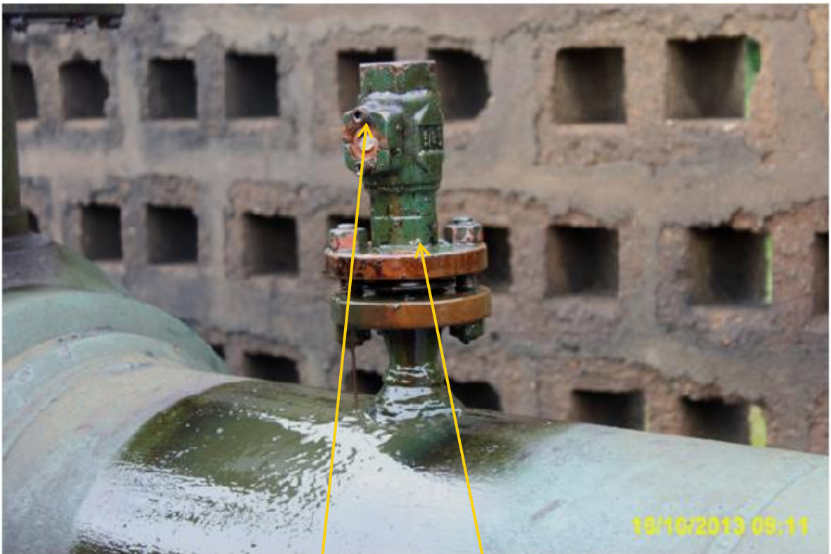
Close up: Positions of tampered valve and missing nuts & bolts on 14" Okordia - Rumuekpe Pipeline riser at Akinima. Picture was taken during Joint Investigation of 16th October 2013.
