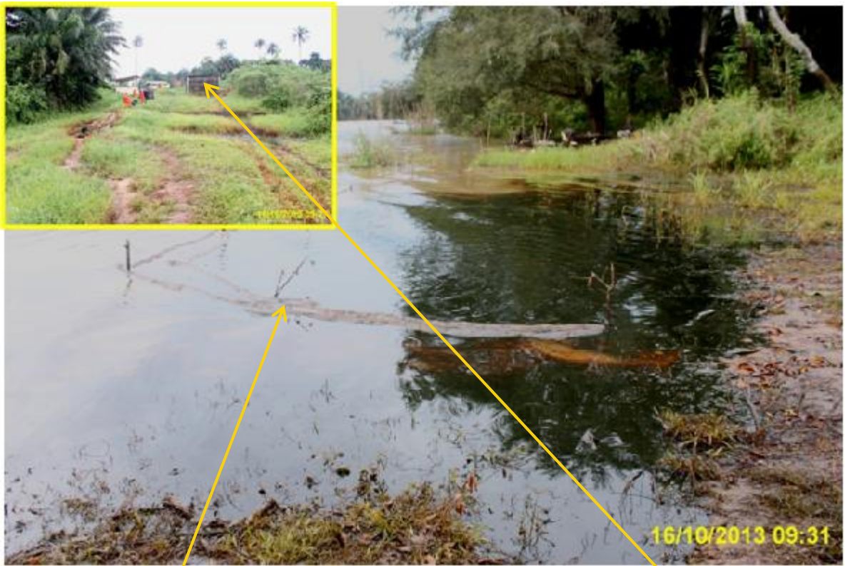
Overview: Parts of spill impact on 14" Okordia - Rumuekpe Pipeline riser at Akinima. Boom in place Picture was taken during Joint Investigation of 16th October 2013.
