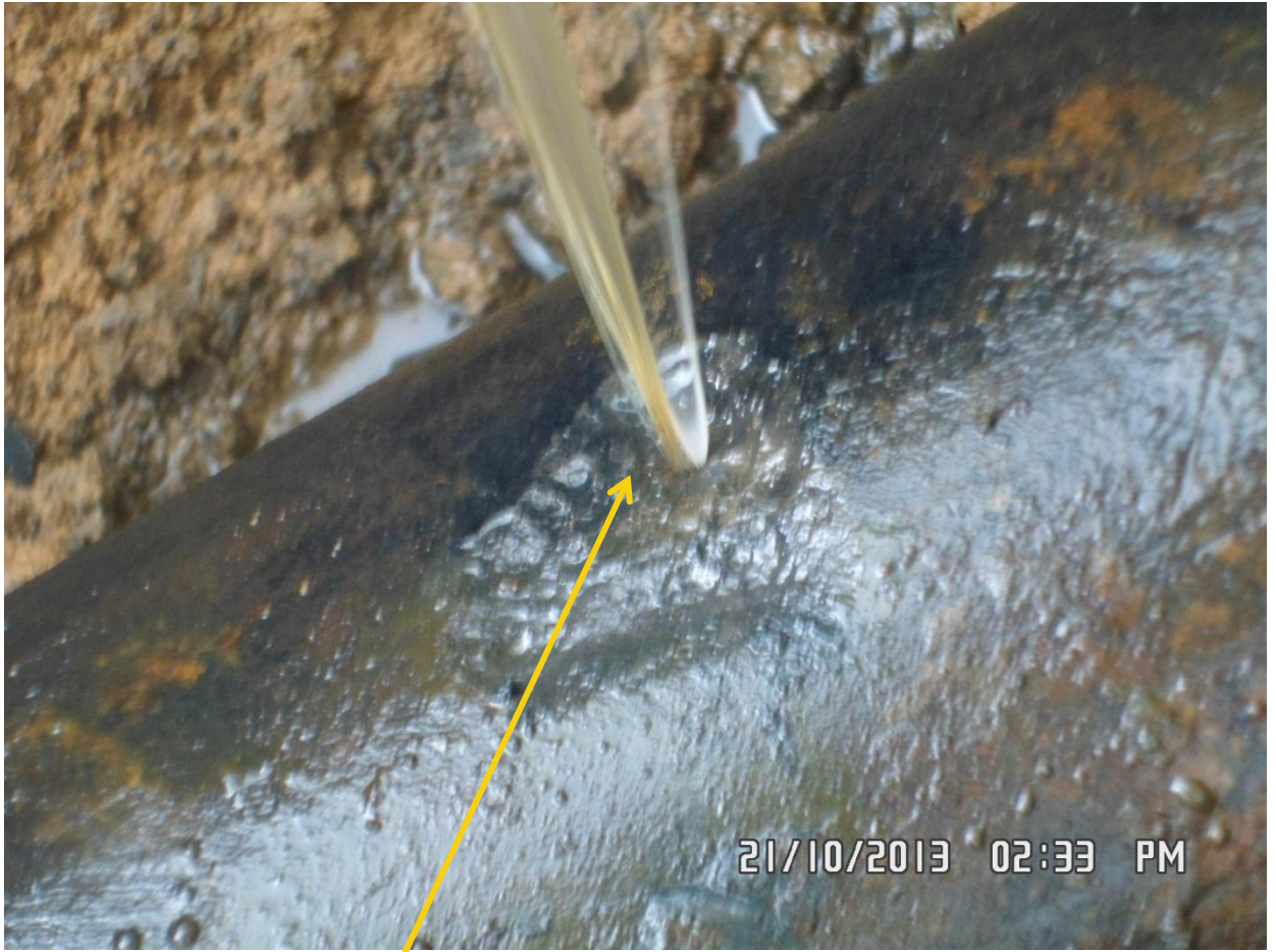
Close-up : Spill due to corrosion on 6" Obigbo-North - Ebubu Pipeline at Obolo. Picture was taken during Joint Investigation of 21st October 2013.
