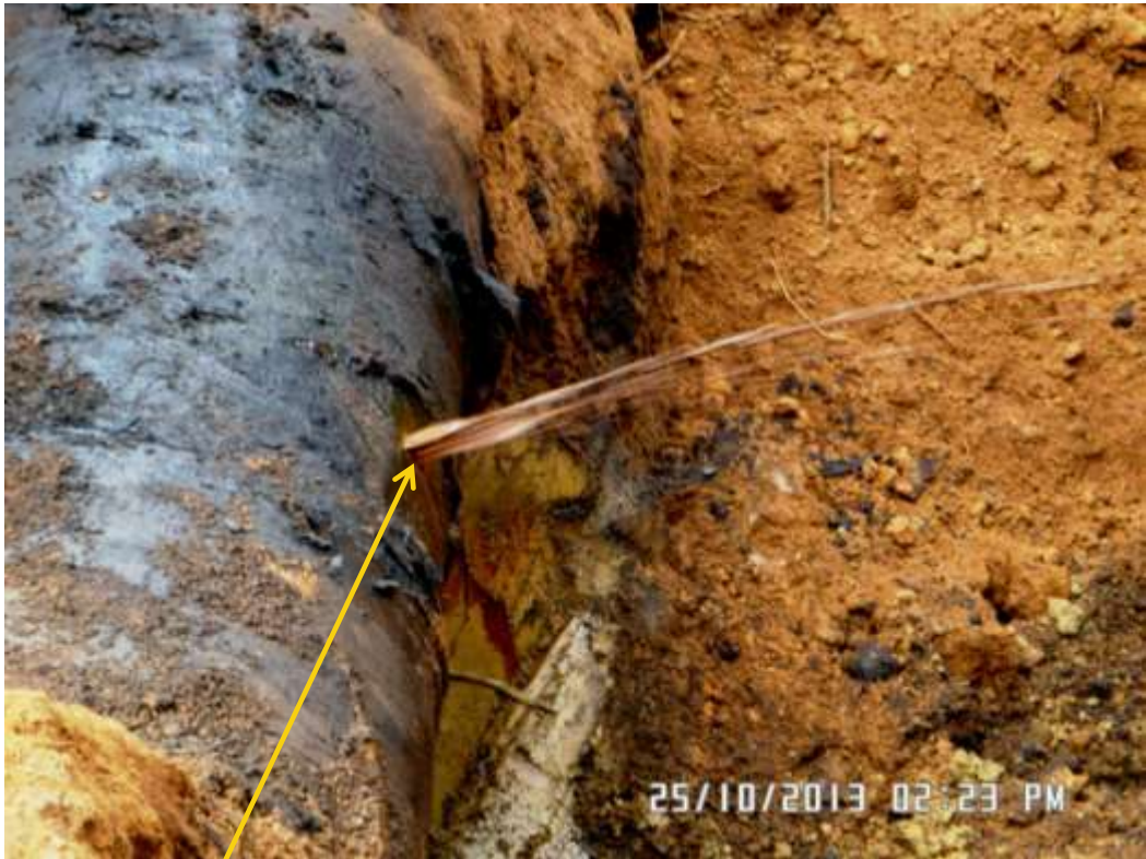
Close-up: Hacksaw cut on 24" Nkpoku - Bomu Trans Niger Pipeline at Biara/Kpите. Picture was taken during Joint Investigation of 25 th October 2013.
