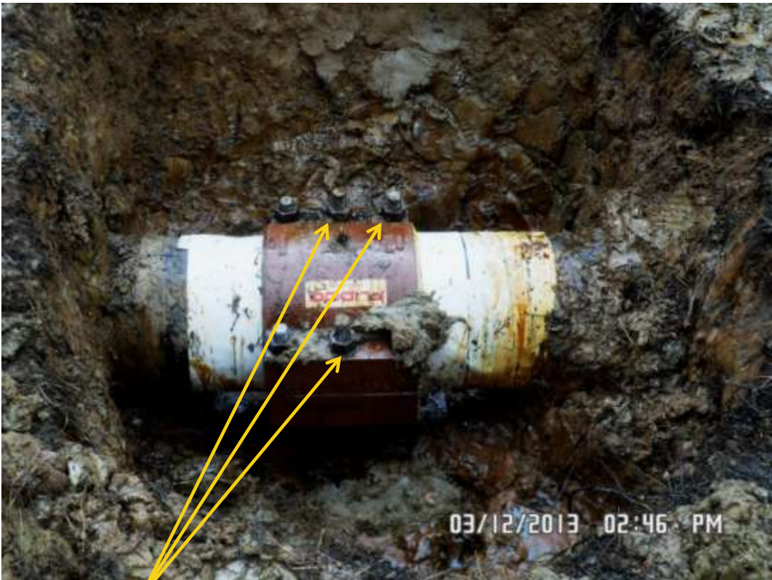
Close-up: Clamp bolts after tightening on 14" Okordia-Rumuekpe Pipeline at Akaramini. Picture was taken during Joint Investigation of 3 rd December 2013.
