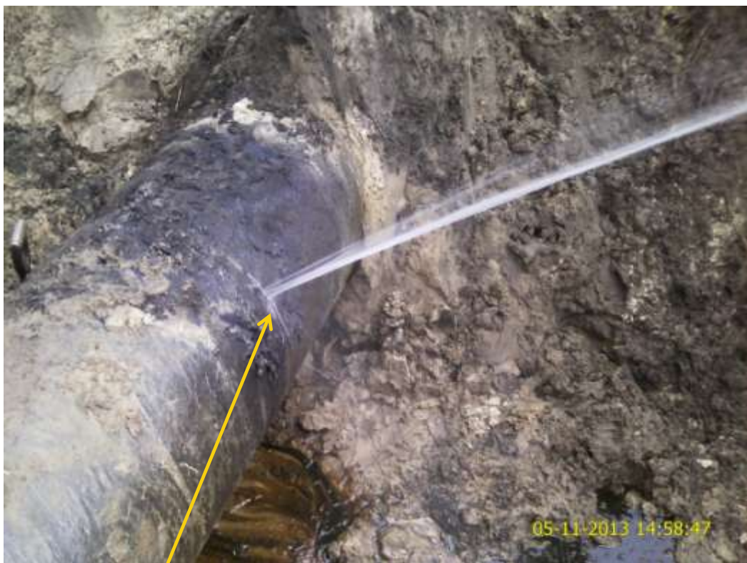
Close-up: Drilled hole/hacksaw cut on 28" Nkpoku-Bomu Pipeline at Gio. Picture was taken during Joint Investigation of 5th November 2013.
