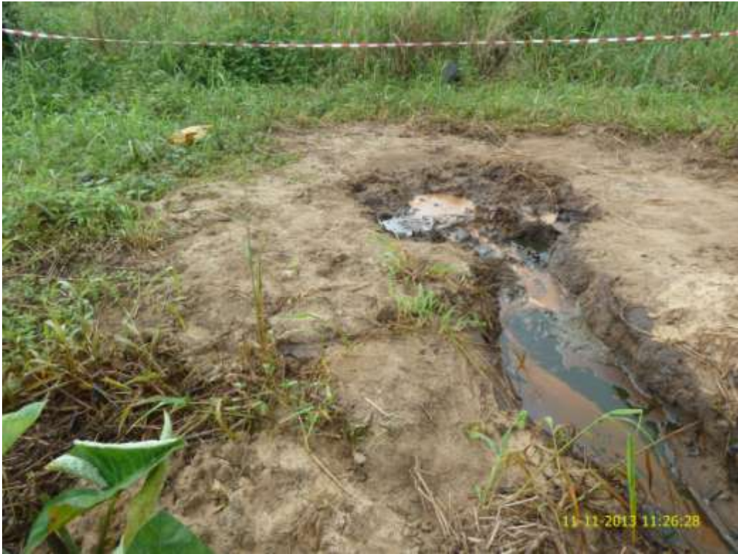
Overview: Part of spill impact on 28" Bomu-Bonny Trans Niger Pipeline right of way at B-dere. Picture was taken during Joint Investigation of 11 th November 2013.
