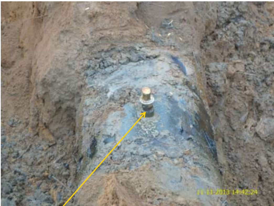
Close-up: Illegal fitting on 28" Bomu-Bonny Trans Niger Pipeline at B-dere. Picture was taken during Joint Investigation of 11 th November 2013.
