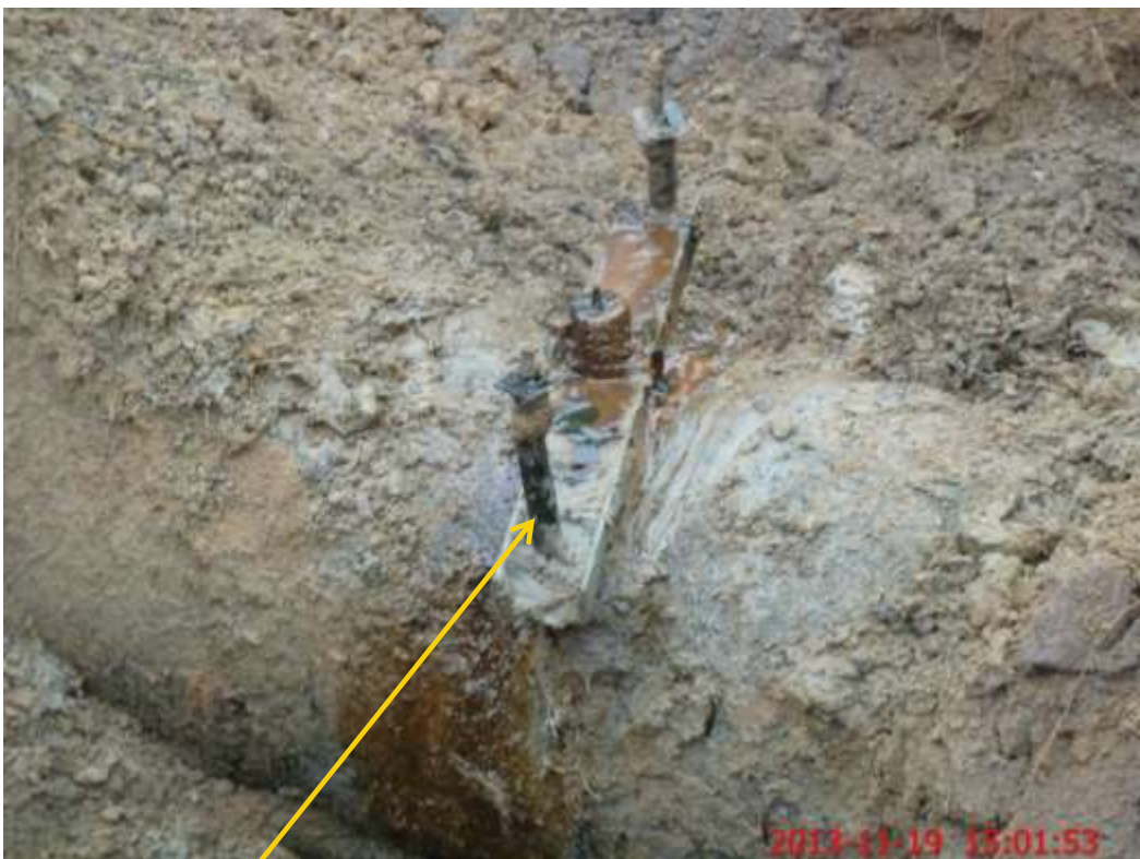
Close-up: Illegal fittings on 24" Nkpoku-Bomu Trans Niger Pipeline at Egbalor. Picture was taken during Joint Investigation of 19th November 2013.
