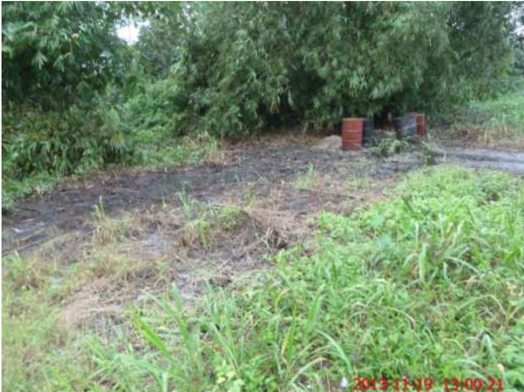
Overview: Part of spill impact on 24" Nkpoku-Bomu Trans Niger Pipeline right of way at Egbalor. Picture was taken during Joint Investigation of 19th November 2013.
