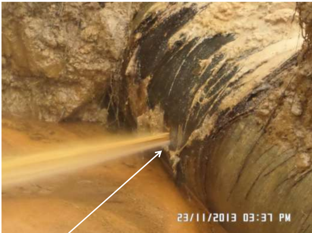
Close-up: Hacksaw cut on 28" Bomu - Bonny Pipeline at Kpor/K-dere. Picture was taken during Joint Investigation of 23 rd November 2013.
