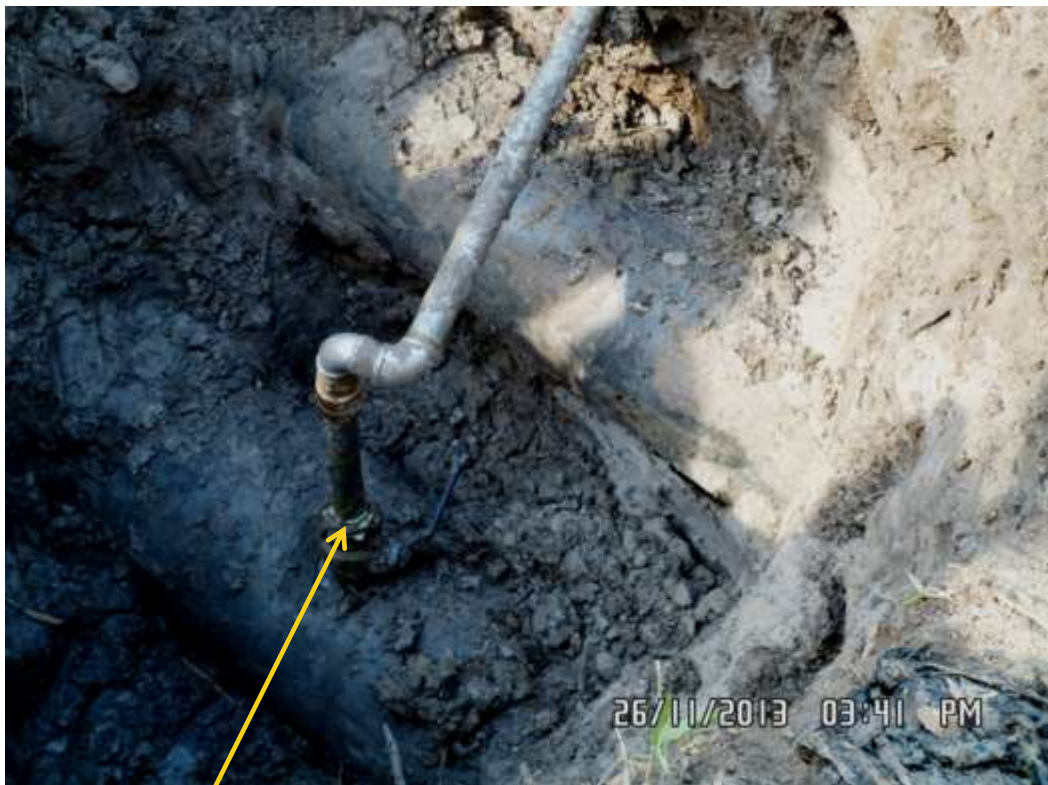
Close-up: Illegal fitting on 14" Okordia-Rumuekpe Pipeline at Imogu. Picture was taken during Joint Investigation of 26 th November 2013.
