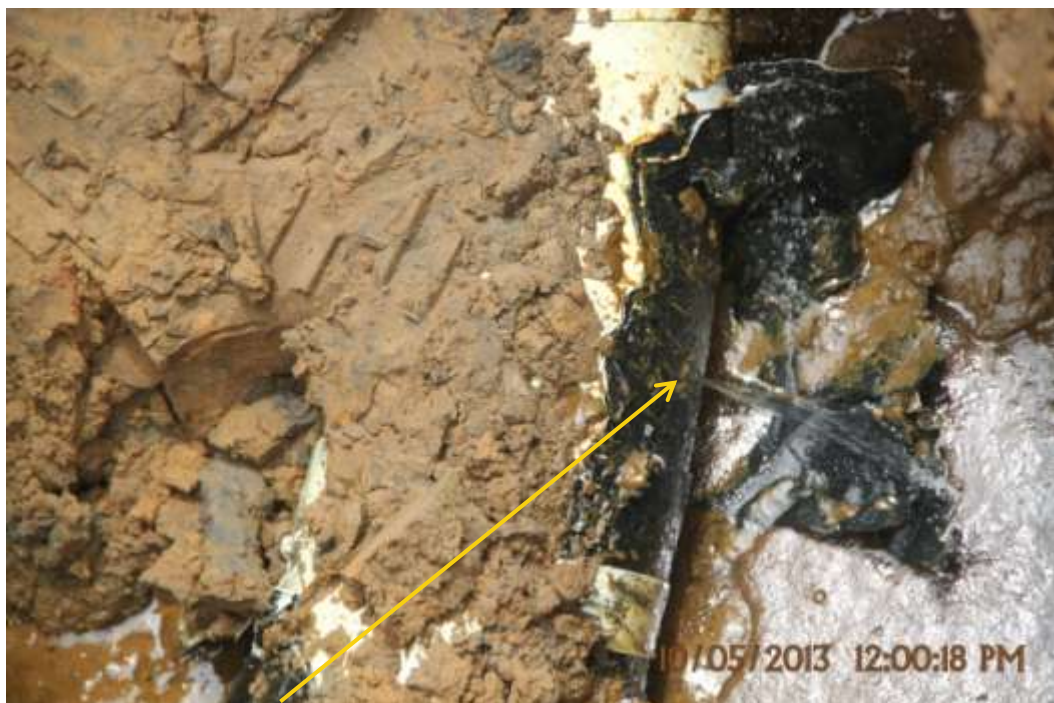
Close up: Leak due to corrosion on Yokri Manifold7 Low Pressure1 line at Sokebolou. Picture was taken during Joint Investigation of 10 th May 2013.
