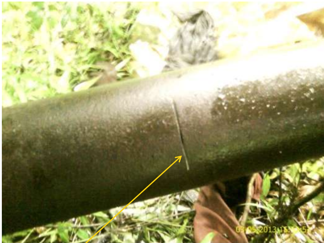
Close up: Hacksaw cut on Adibawa NorthEast Well1L flowline at Biseni. Picture was taken during Joint Investigation of 3 rd May 2013.
