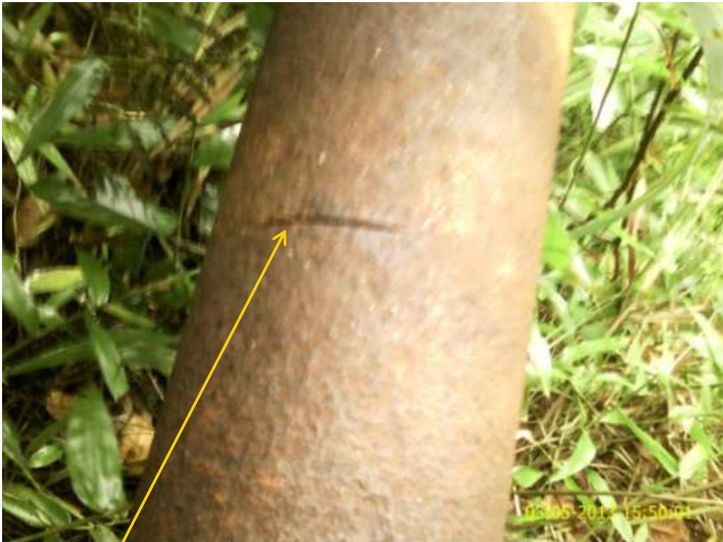
Close up: Hacksaw cut on Adibawa NorthEast Well1L flowline at Biseni. Picture was taken during Joint Investigation of 3 rd May 2013.
