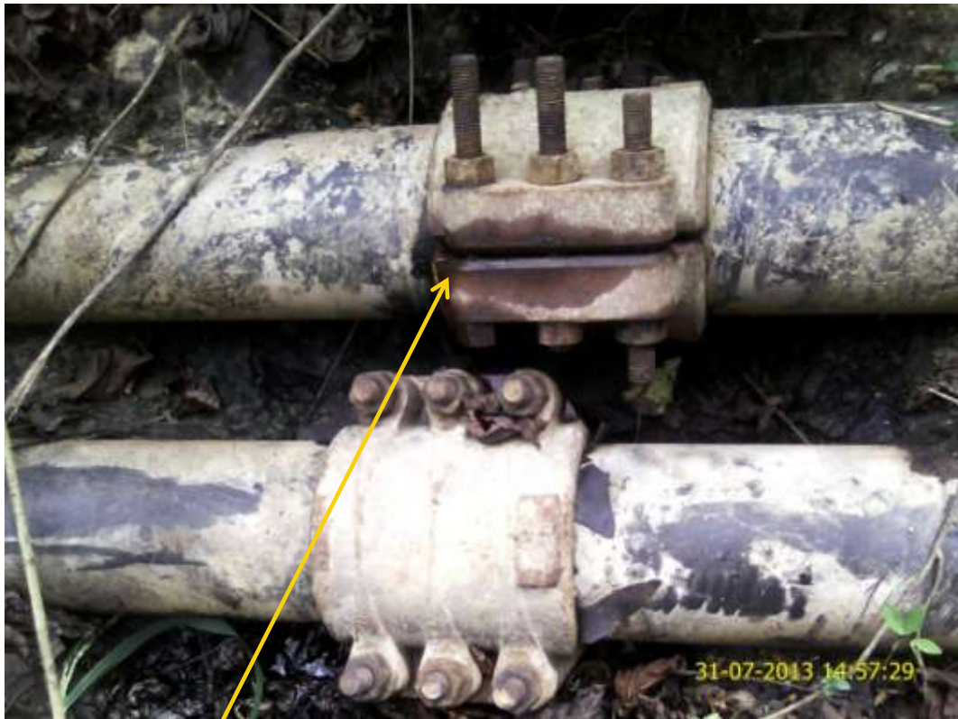
Close-up : Spill point on 6" Adibawa NorthEast Flowline at Biseni. Picture was taken during Joint Investigation of 31 st July 2013.
