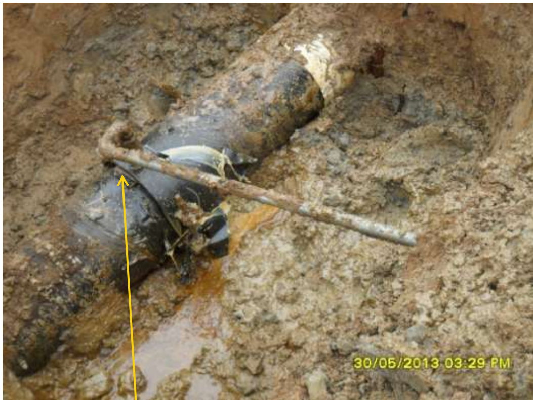
Close up: Illegal fitting on 12" Imo River2 pipeline at Umuedeokwara. Picture was taken during Joint Investigation of 30 th May 2013.
