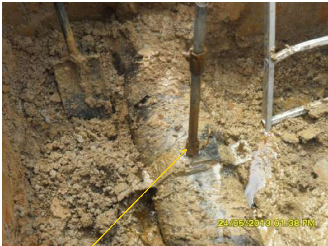
Close up: Illegal fitting on 12" Imo River2 pipeline at Umuedeokwara. Picture was taken during Joint Investigation of 24 th May 2013.
