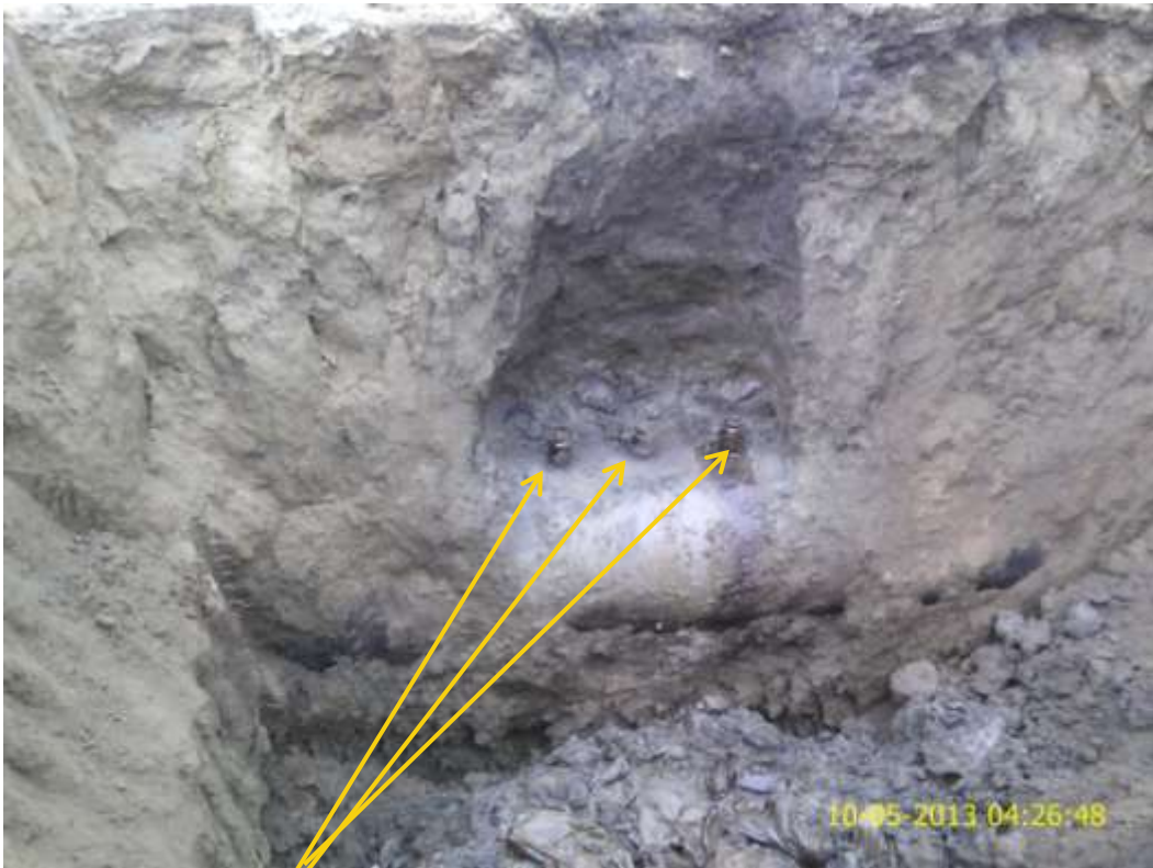
Close up: Illegal fittings on 36" Nkpoku-Bomu pipeline at Elenwo. Picture was taken during Joint Investigation of 10 th May 2013.
