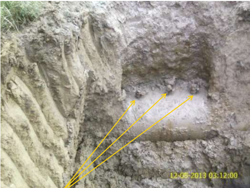
Close up: Illegal fittings on 36" Nkpoku-Bomu pipeline at Eelenwo. Picture was taken during Joint Investigation of 12 th May 2013.
