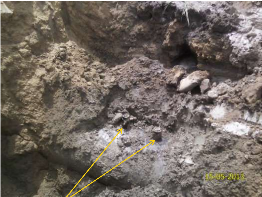
Close up : Illegal fittings on 36" Nkpoku-Bomu pipeline at Akpajo. Picture was taken during Joint Investigation of 15 th May 2013.
