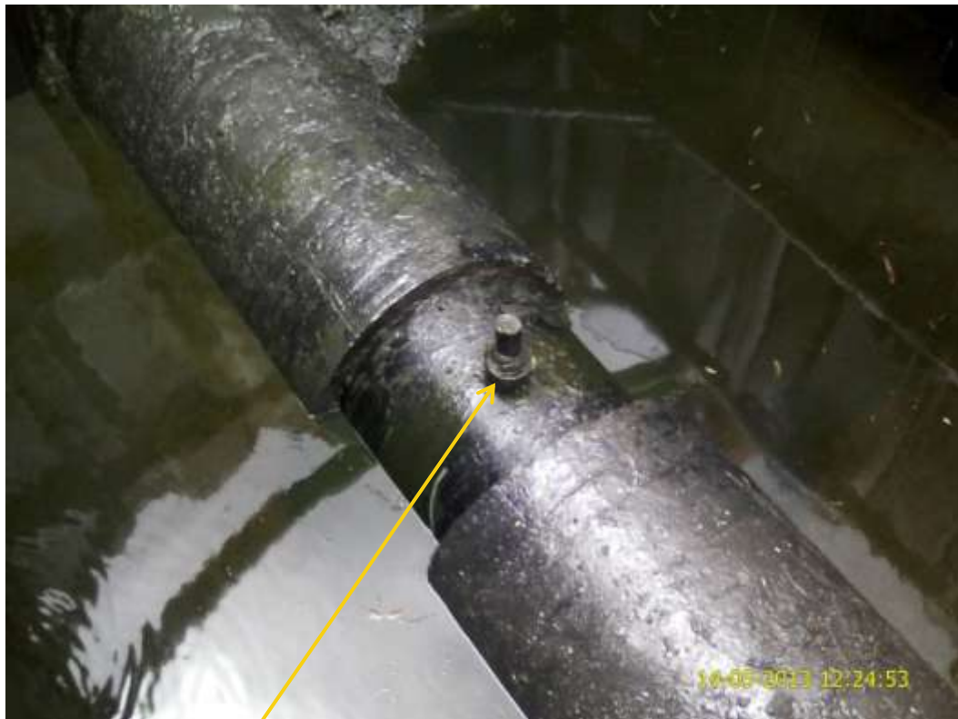
Close up: Illegal fitting on 30" Nembe Creek pipeline at Boro (Kula). Picture was taken during Joint Investigation of 14 th May 2013.
