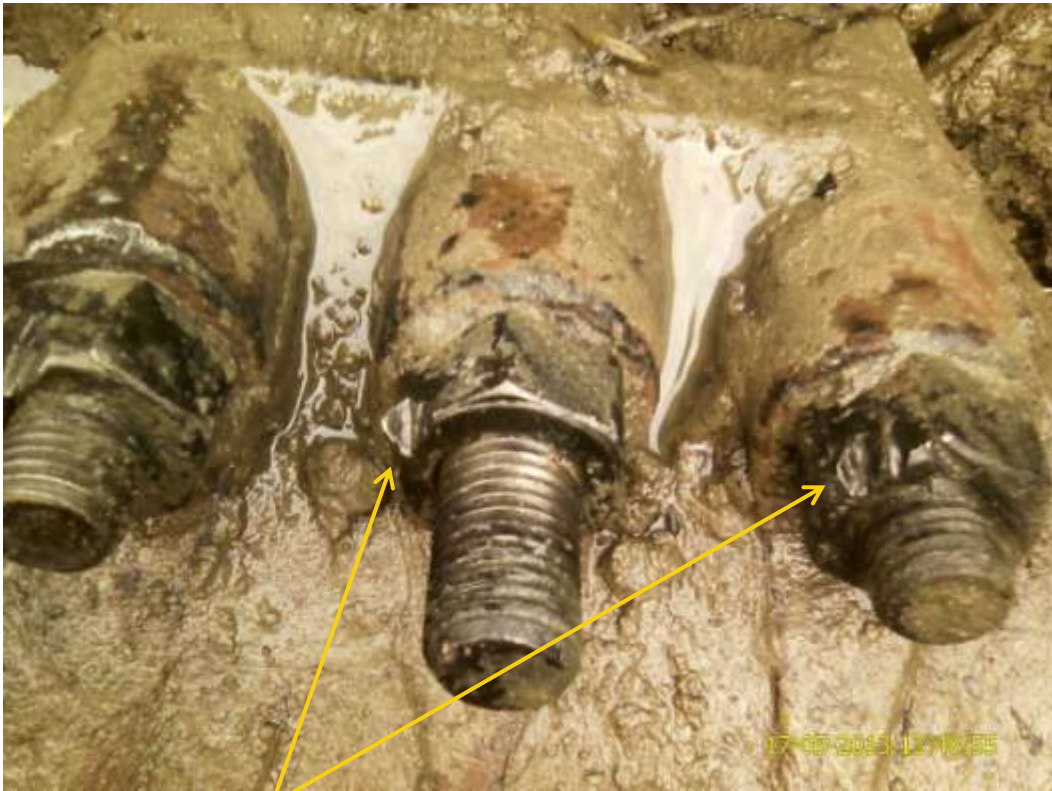
Close up: Chisel marks on clamp nuts on 8" Ubie-Ukpeliede pipeline at Idu-Ekpeye . Picture was taken during Joint Investigation of 17 th May 2013.
