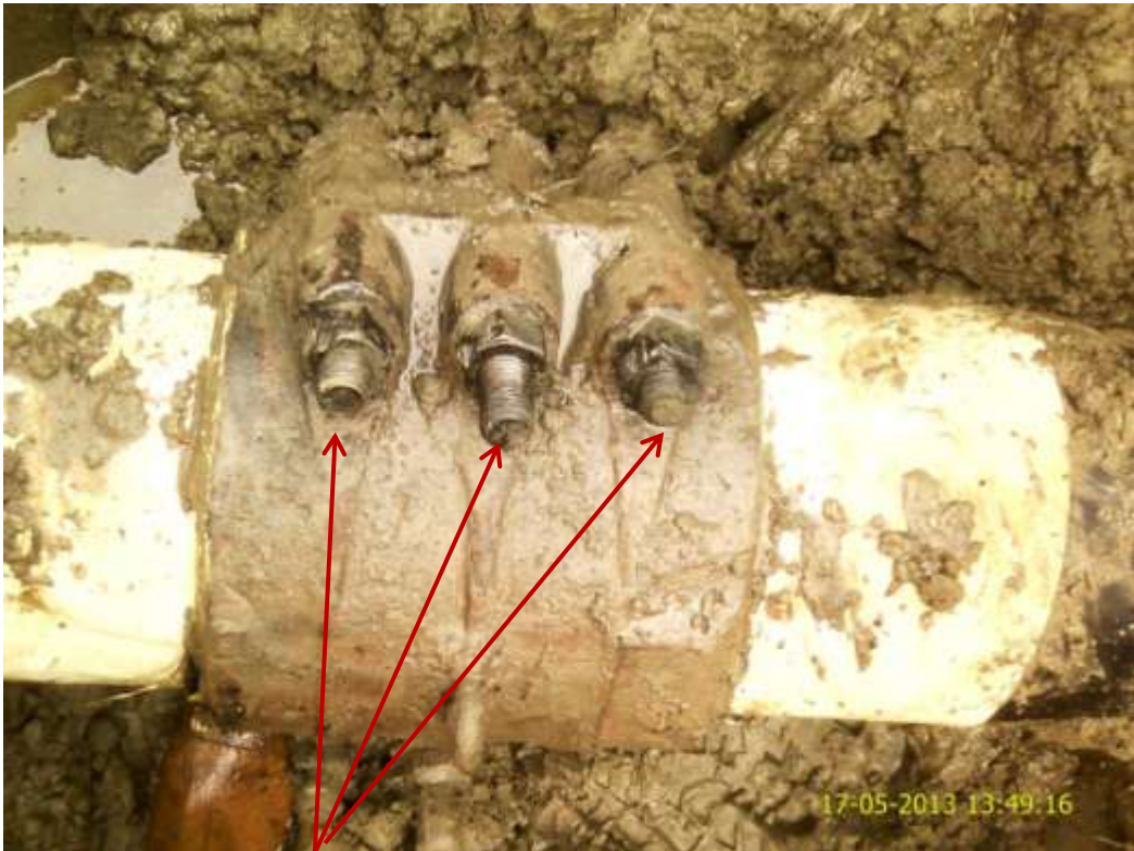
Close up: Chiseled clamp nuts on 8" Ubie-Ukpeliede pipeline at Idu-Ekpeye . Picture was taken during Joint Investigation of 17 th May 2013.
