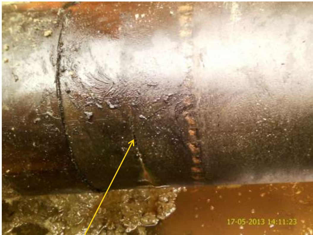
Close up: Hacksaw cut on 8" Ubie-Ukpeliede pipeline at Idu-Ekpeye . Picture was taken during Joint Investigation of 17 th May 2013.
