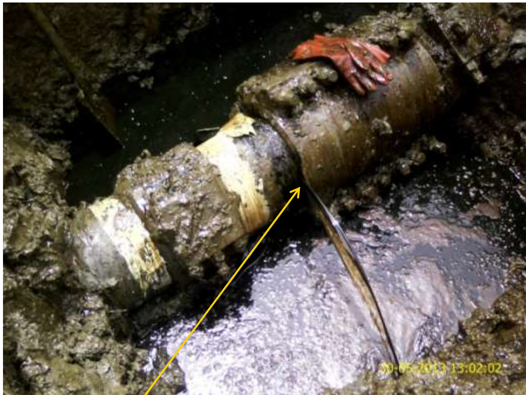
Close up: Spill due to hacksaw cut on 12" Adibawa-Okordia pipeline at Ikarama. Picture was taken during Joint Investigation of 30 th May 2013.
