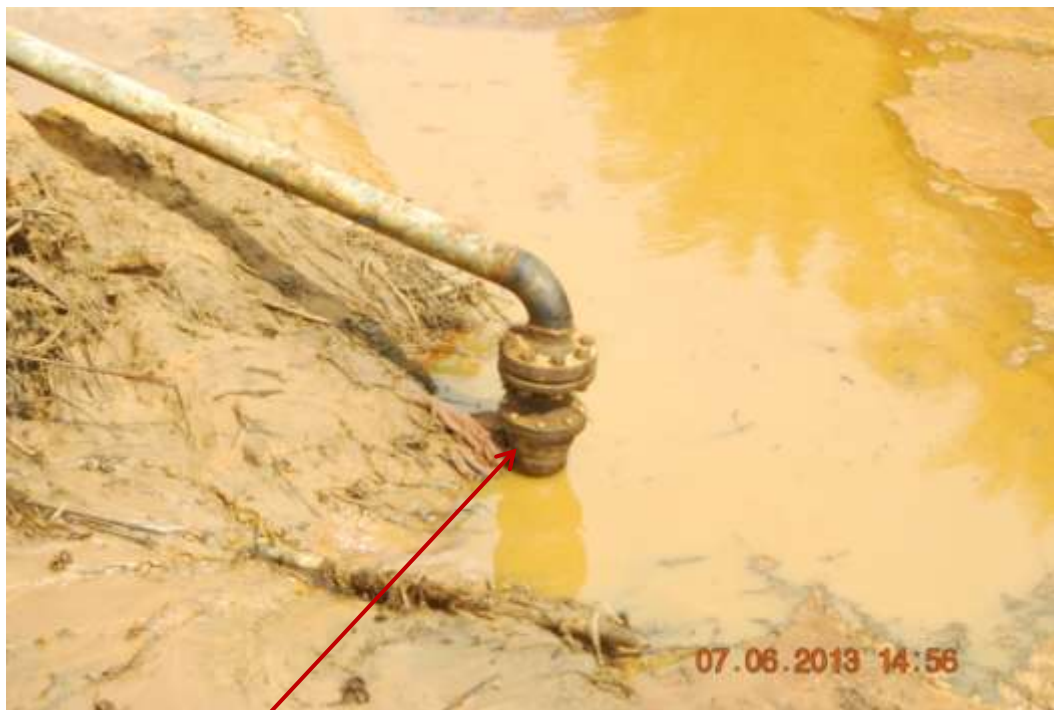
Close up: Illegal fitting on 20" Otumara-Escravos trunkline at Ugbokodo. Picture was taken during Joint Investigation of 7 th June 2013.
