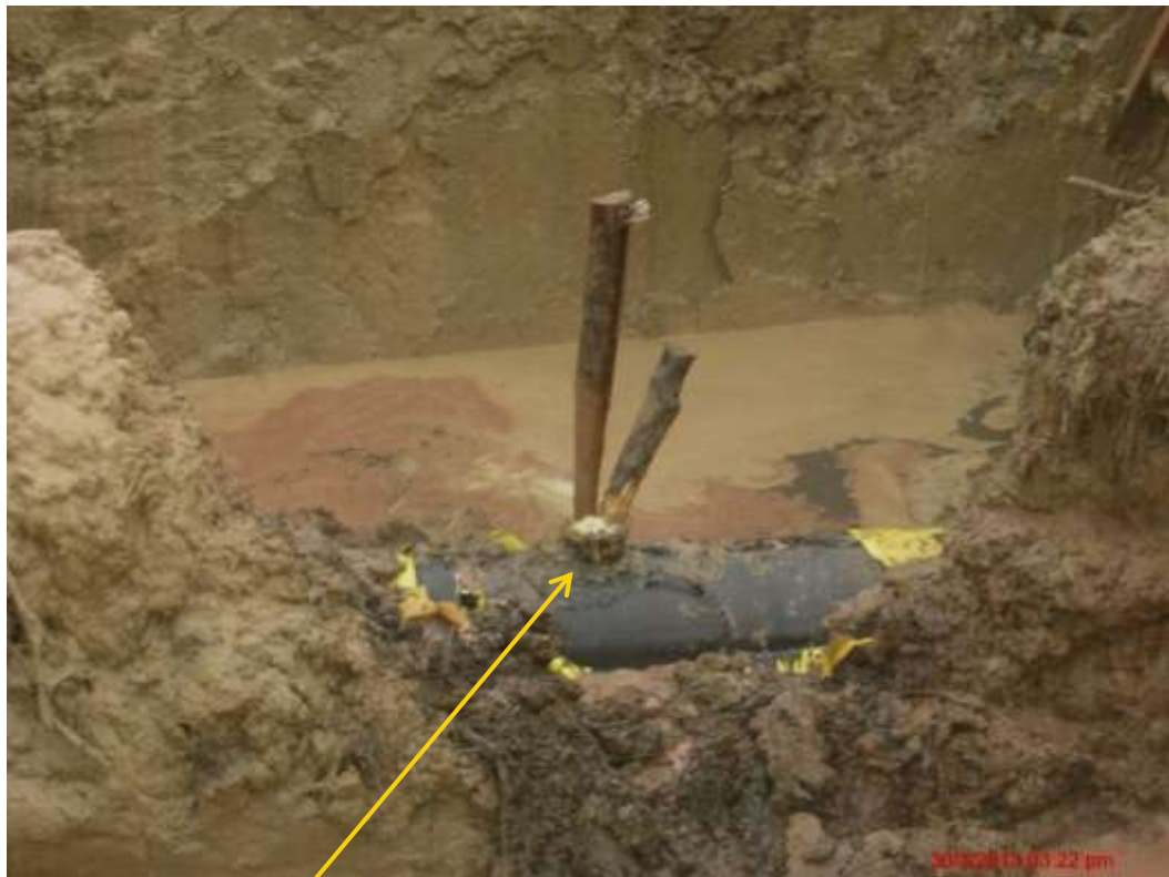
Close up: Illegal fitting on 12" Imo River2 – Ogale pipeline at KomKom. Picture was taken during Joint Investigation of 30 th March 2013.
