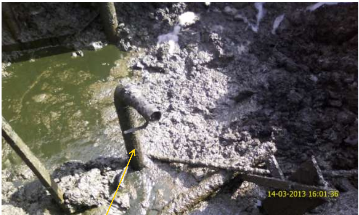
Close up: Illegal fitting on 30" Nembe Creek pipeline at Bille. Picture was taken during Joint Investigation of 14 th March 2013.
