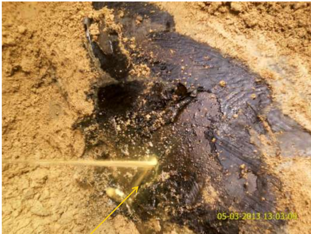
Close up: Hacksaw cut on 8" Assa-Rumuekpe pipeline at Awara. Picture was taken during Joint Investigation of 5 th March 2013.
