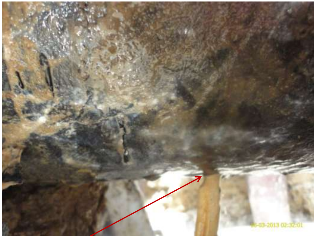
Close up: Location of corrosion point on 14" Okordia-Rumuekpe pipeline at Ikarama. Picture was taken during Joint Investigation of 16 th March 2013.
