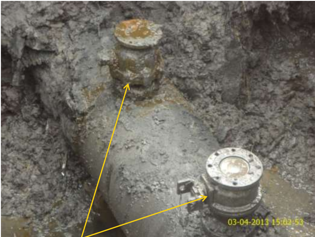
Close up: Illegal fittings on 24" Nembe Creek Trunkline at Aberedo-A. Picture was taken during Joint Investigation of 3 rd April 2013.
