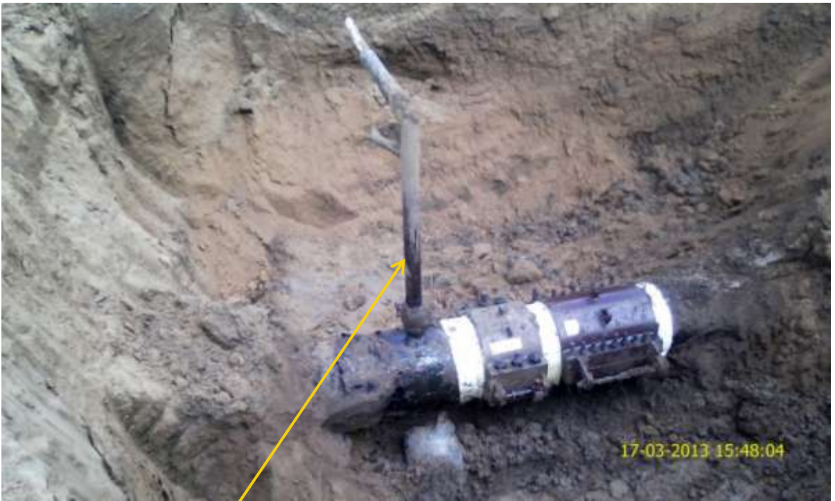
Close up: Illegal fitting on 18" Assa-Rumuekpe pipeline at Egbeda. Picture was taken during Joint Investigation of 17 th March 2013.
