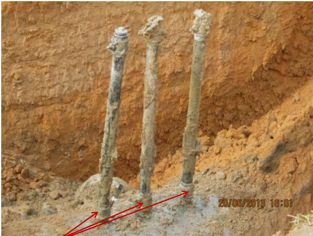
Close up: Illegal fittings on 36" Rumuekpe-Nkpoku Trans Niger pipeline at Aluu. Picture was taken during Joint Investigation of 20 th June 2013.
