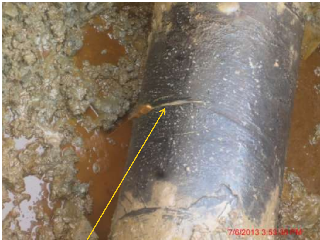
Close up: Hacksaw cut on 14" Okordia-Rumuekpe pipeline at Ikarama. Picture was taken during Joint Investigation of 7 th June 2013.
