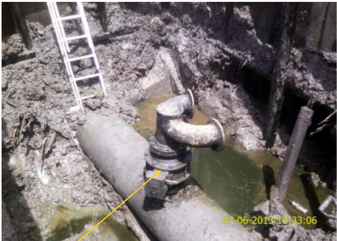
Close up: Illegal fitting 24" Nembe Creek pipeline at Adamakiri. Picture was taken during Joint Investigation of 7 th June 2013.
